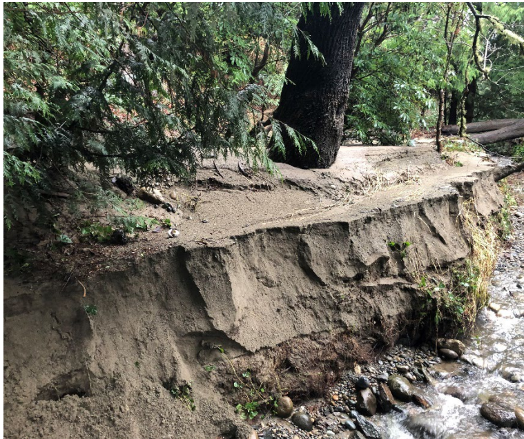
A portion of the heavily impacted Perrinville Creek is showing impacts from extreme sediment loads during storm events; the City has announced a major restoration project will be kicking off for this drainage basin.
