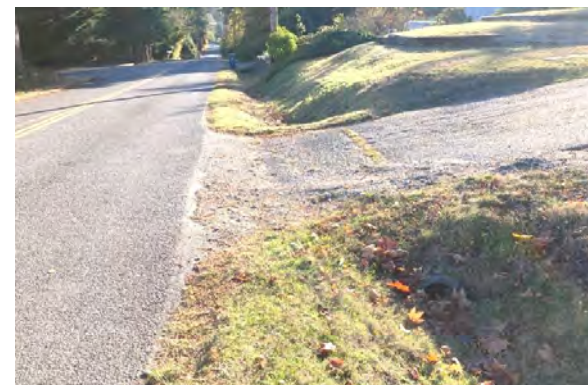
Existing stormwater drainage ditches in the ROW could be retrofitted to provide water quality treatment and infiltration.
