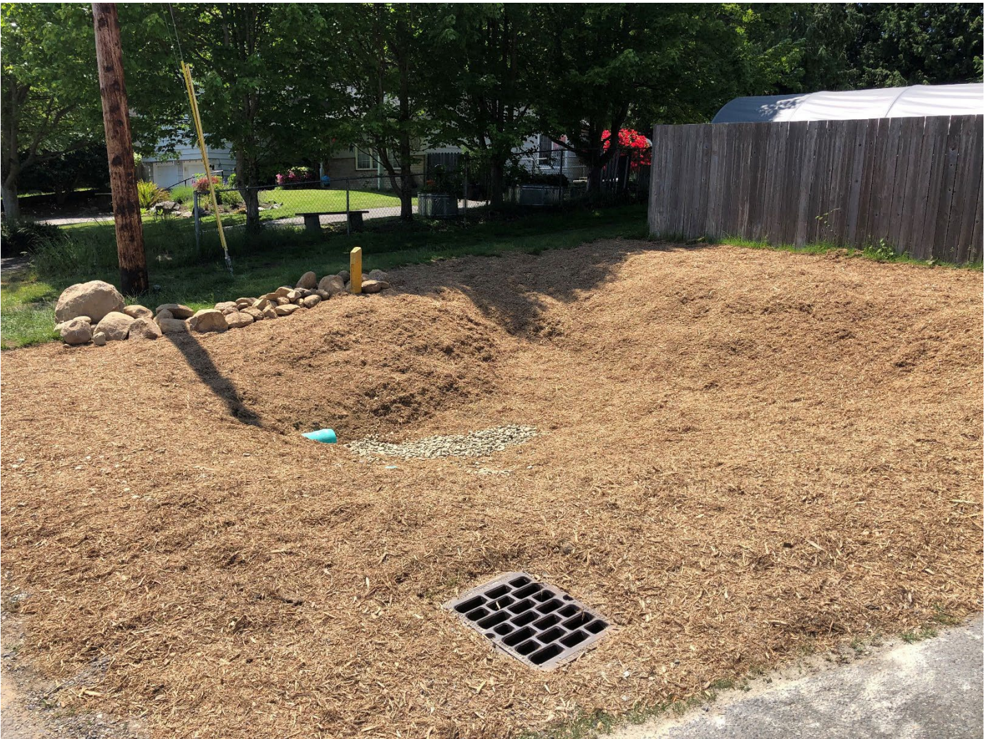
As the contractor, Snohomish Conservation District (SCD) excavated a large unused piece of land, where it was converted to a useful and beneficial rain garden. [Photo taken June 1, 2023]
